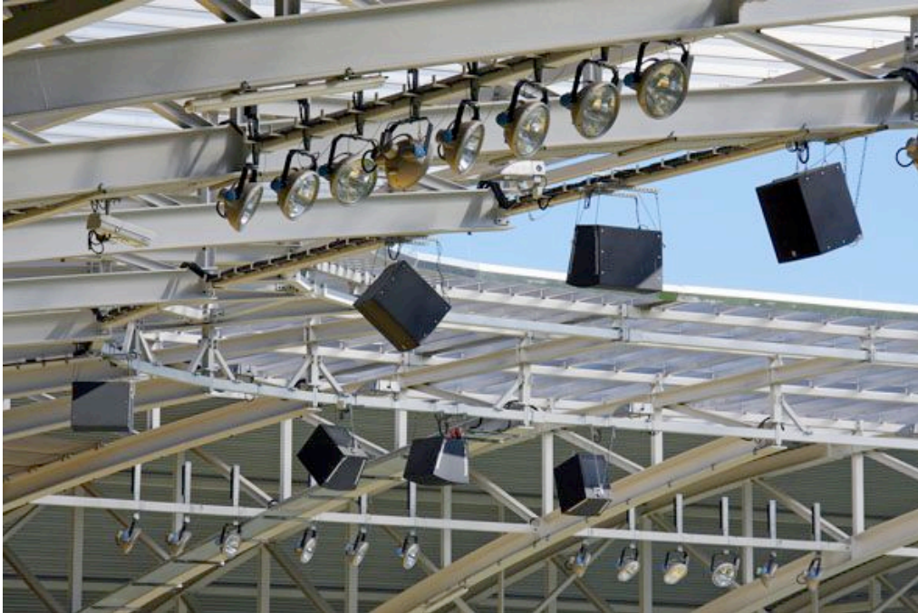
Providing sound reinforcement for the largest single-tier stadium in Germany: Electro-Voice FRX-PI series loudspeakers
